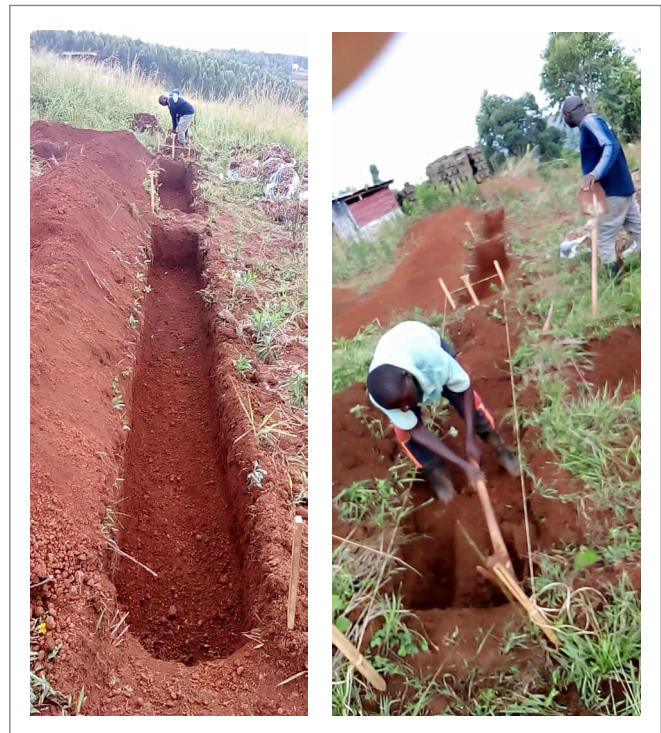
The Fanya Juu Method of Rain Water Harvesting on A Contour Line
